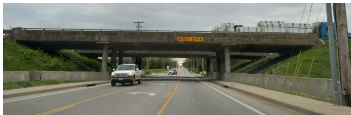
Narrow sidewalks under I-44 like those shown at National Avenue impede connectivity and create safety concerns.
